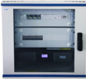
AE CGLine+ System inkl. Notstromversorgung
